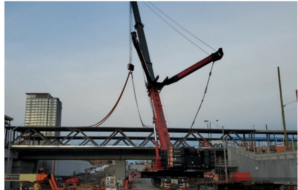
The pedestrian bridges run parallel to the new rail bridge. (Metrolinx photo)
